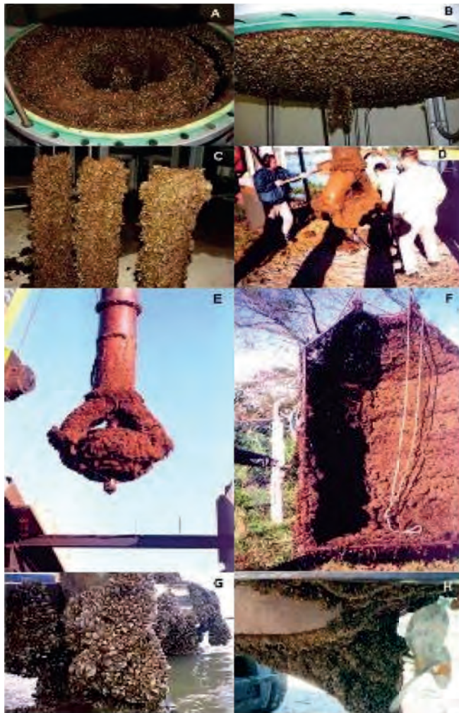
Figure 5. Artificial substrates used by Limnoperna fortunei : 3A, clogged self-cleaning filter; 3B, detail of the lid; 3C, cylinders inside the same filter; 3D, beginning of the cleaning process of a pump collecting encrusted water; 3E, pump hoisted by crane from the roof; 3F, pump protective grid; 3G, marina pier; 3H, hull of a boat used for fishing in Lake Guaíba and Lagoa dos Patos, being transported by road to another source, posing a risk of contamination. Photos: A, B, C: Gustavo Darrigran, www.malacologia.com.ar ; D, E, F: José Imada, CORSAN; G: Augusto Chagas: Biociências , 2004, 13(1); H: MCD Mansur: Brazilian Magazine of Zoology 2003, 20(1). Source: Santos et al. (2012a).
