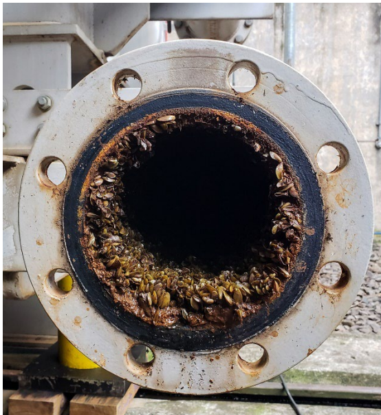
Golden Mussels colonizing a water pipe at a hydroelectric plant in Brazil (Moutinho, 2021).
